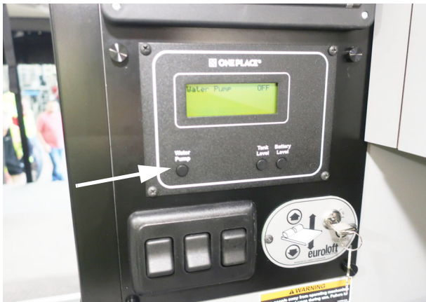
Water pump switch location on Systems Monitor Panel -Typical view
