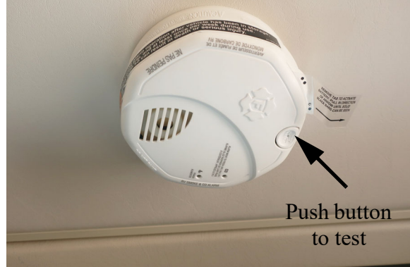
Smoke/carbon monoxide alarm. -Typical View
