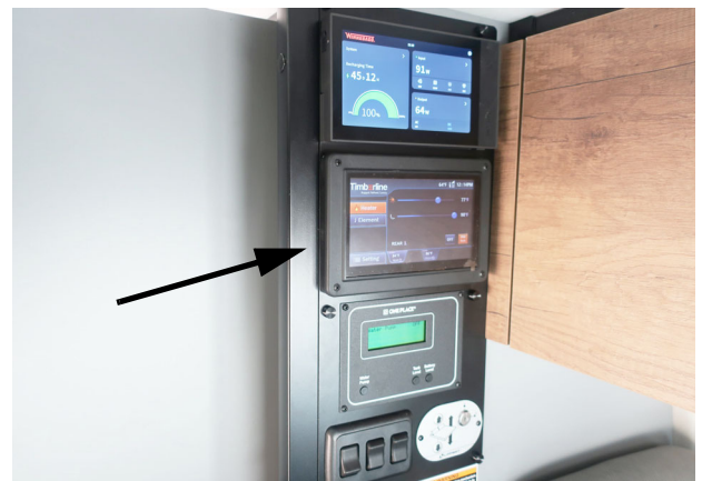
Hydronic Heating System (Located on the monitor panel) -Typical View
