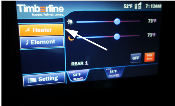
Water heater controls on Systems Monitor Panel -Typical view
