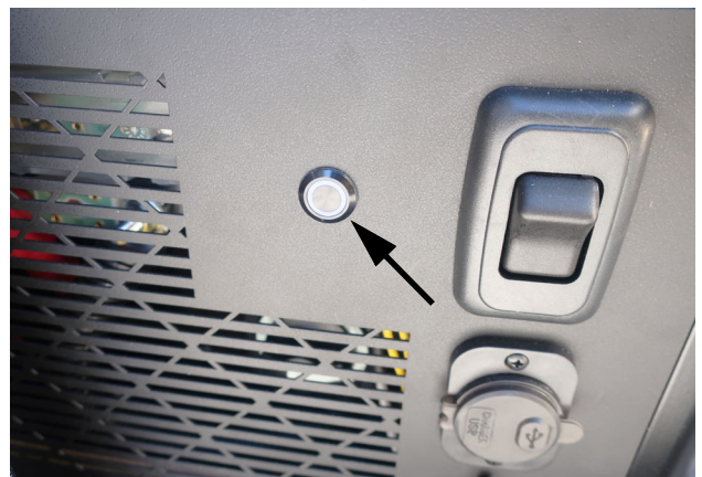
House/Coach Battery Power Controls (Located behind the driver's side rear door). -Typical View
