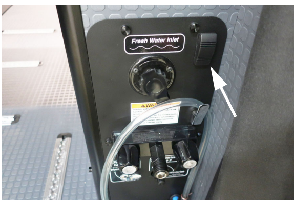
Water pump switch location on Water Center Panel -Typical view
