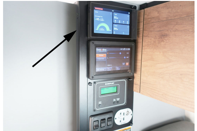
EcoFlow Control Panel (Located on monitor panel) -Typical View
