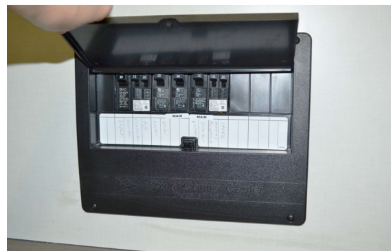
120-Volt Circuit Breakers -Typical View
